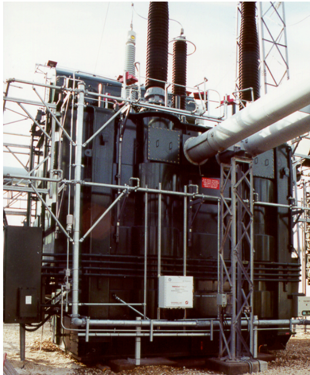
Figure 8 – Fiber optic temperature sensor on a 107MVA converter transformer
